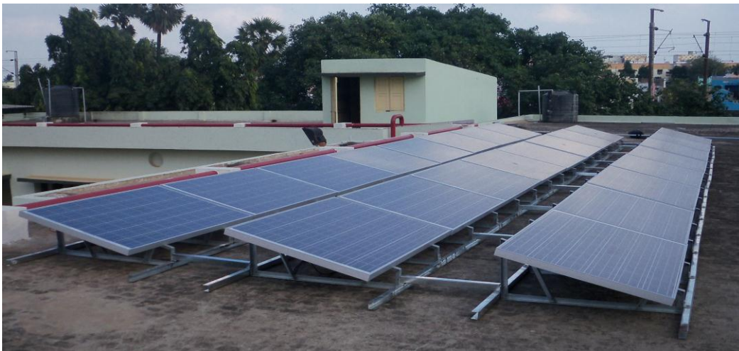
Fig. 5.4 Solar panels placed on roof-top
