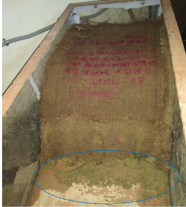
Fig 4.9.2: Soil erosion with using jute mats
