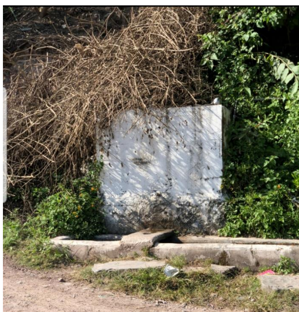
Fig. 4.3: Storage tank of Chauvsa
