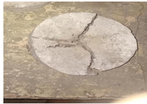
Crack failure at 0.5%
