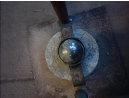
Crack initiation at 1.5%
