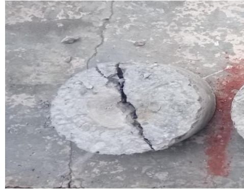
Crack failure at 0%
