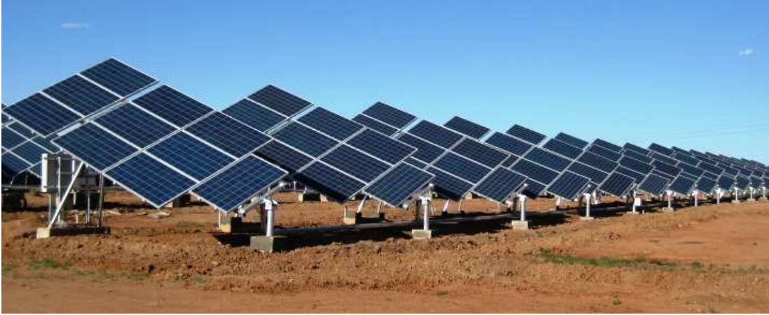
Figure 3.2: Tilted single axis tracker in Siziwangqi, China
