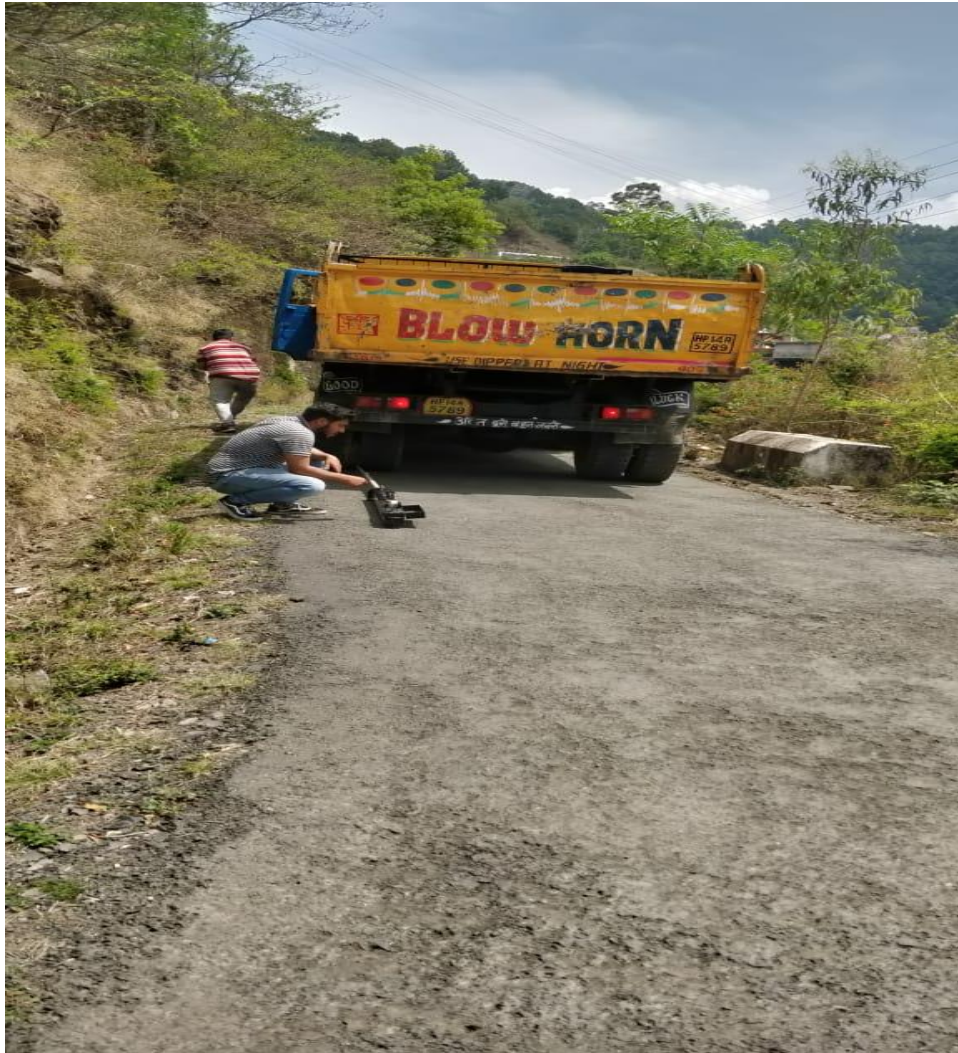
Fig. 4.7 Road condition of RR2
