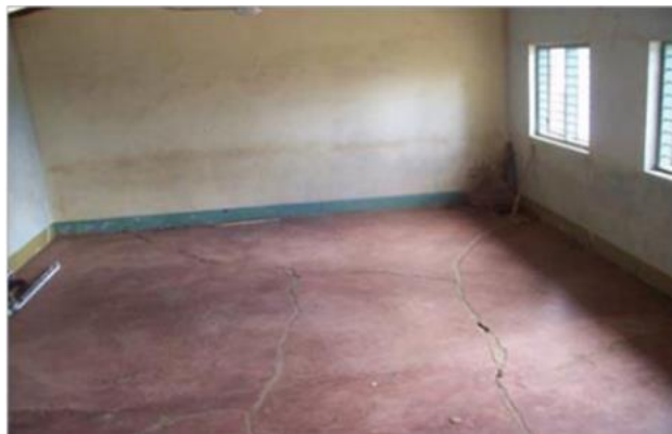
(b): Heaving of interior floor causing cracking of slab
