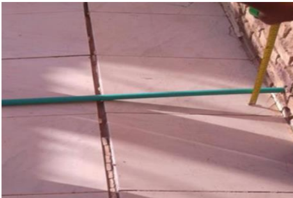
Fig 1.3 (a): Heaving of interior floor causing cracking of floor tiles
