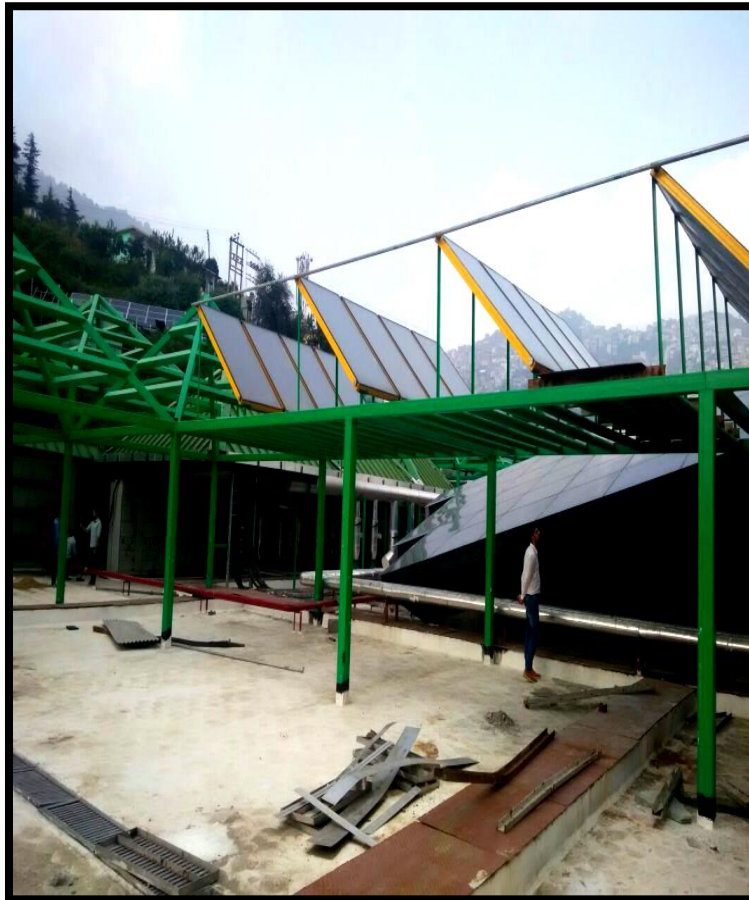
Fig. 12 On roof 'Collector Drain Pipes' are there which are attached to 'Rain Water Harvesting pit' at the ground
