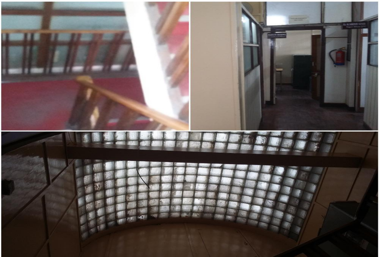
Figure 4: Solarium installed inside the himurja complex & internal office space
