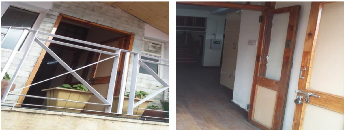
Figure 2: Double Door system for proper ventilation and temperature maintenance
