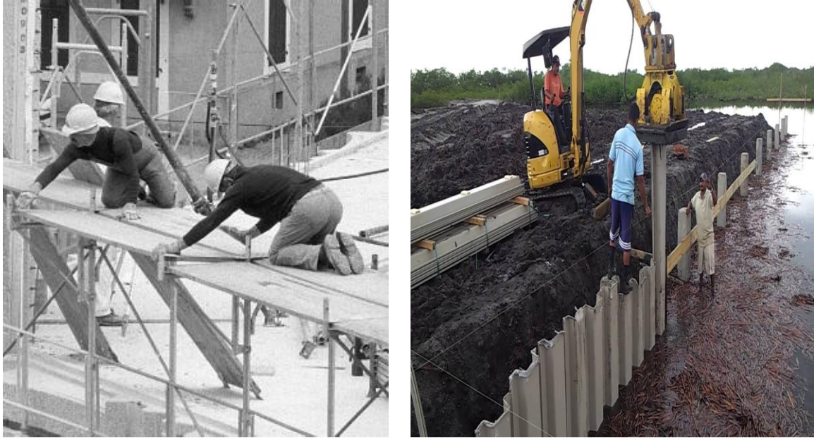
Figure3.3 (a) Workers working a height[26] Figure3.3 (b) Striking of worker with vehicle
