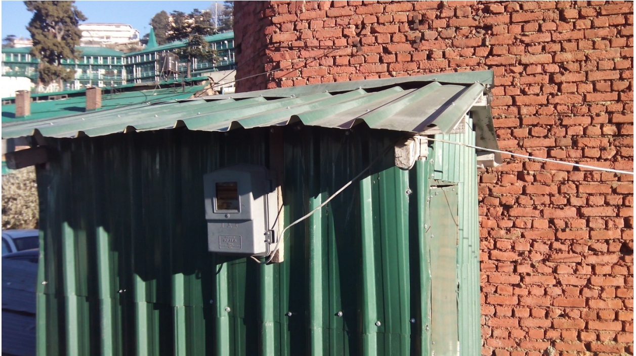
Figure 16 Monitoring station-2 at “Old ISBT”.
