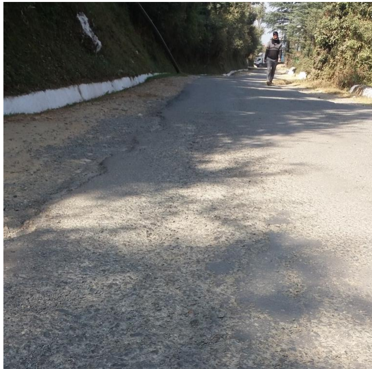
Fig. 1. 1 Flexible pavement having roughness
