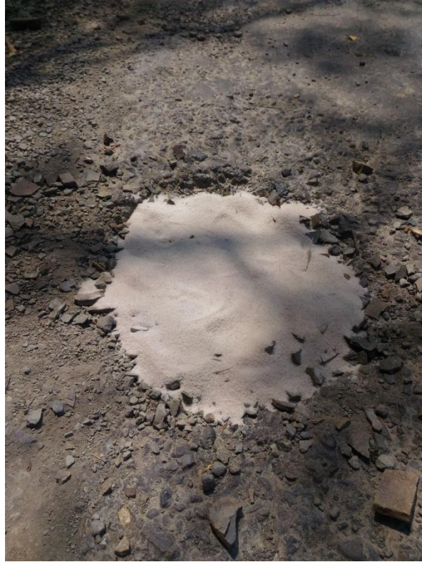
Fig. 4. 5 Measurement of pothole
