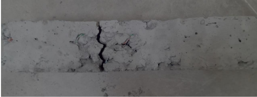
Fig. 4.29 Cracks in DFCMS beam
