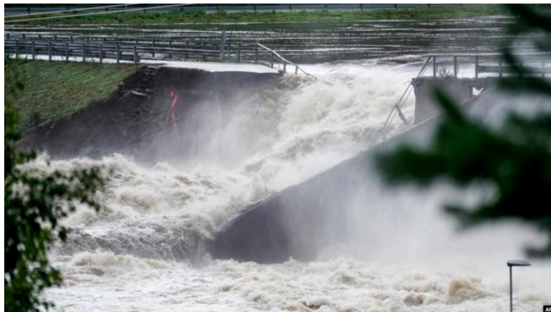
Fig 1.14: Heavy rain cause partial collapse of Norwegian dam
