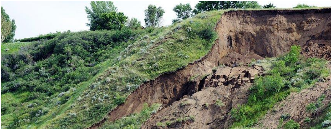
Figure 1.1 Soil slope failure
