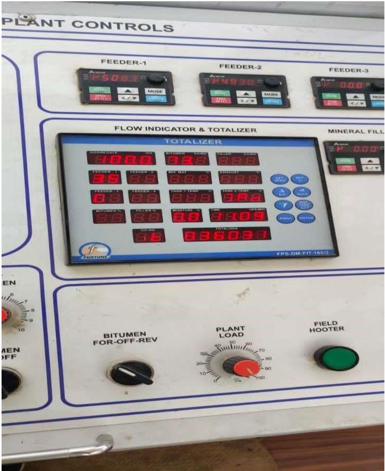
Figure 3.1: Control panel of batching plant
